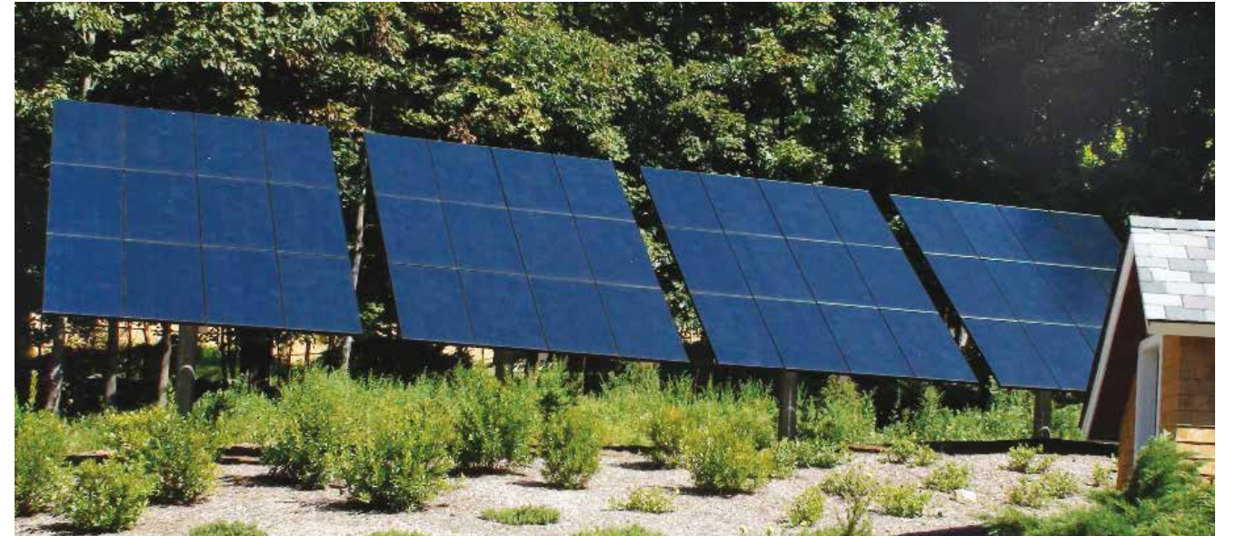
Nearly Off-Grid. Fourteen photovoltaic panels power the house, while an additional set in the backyard provides heating for the pool. Overall, 94.2% of the home’s energy needs are met by solar technologies.
