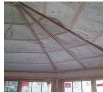
Double Insulated. Crews insulated the precast concrete walls with 1” of rigid foam board followed by spray foam.
